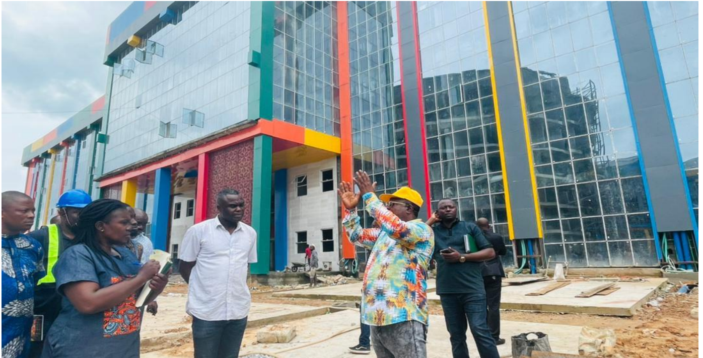
Figure 33. His Excellency Engr. David Umahi inspecting progress of work during the construction of the University buildings
